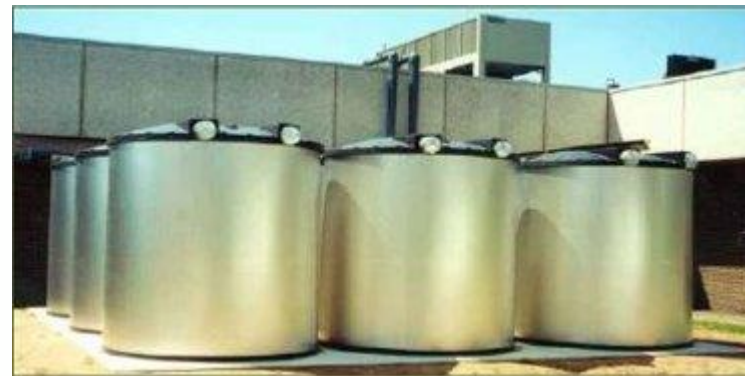
Chilled Water Storage
